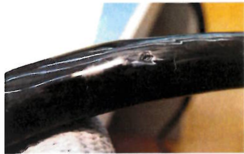
Figure 8: Damaged Motor Cable
