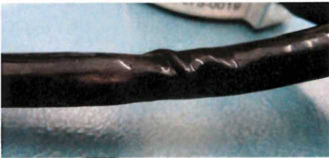
Figure 7: Damaged Motor Cable
